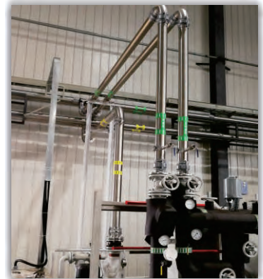
● Oil and Cooling water for Machinery
