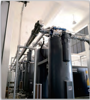
● Compressed Air for Foods
