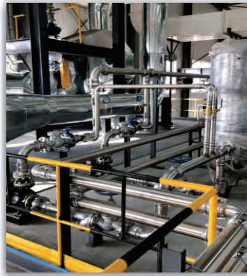
● Cooling water for new Material
