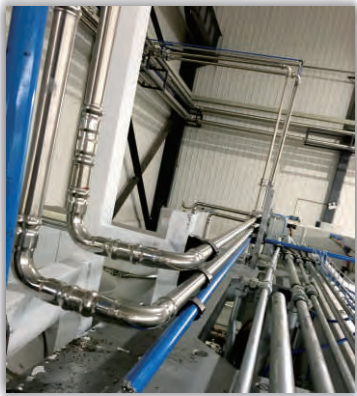
● Cooling water for Auto Parts.
